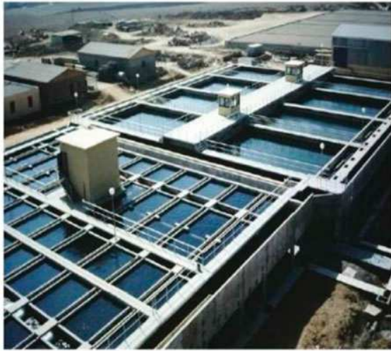
Fig. 5. Pulsa tube clarifier.
