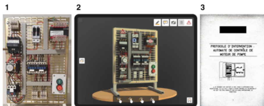
Fig. 2. From left to right: 1. The electrical panel on which the maintenance operation is to be performed. 2. The telecollaboration application on the Tab S7 + 5G tablet. 3. The manual detailing the maintenance procedure.
