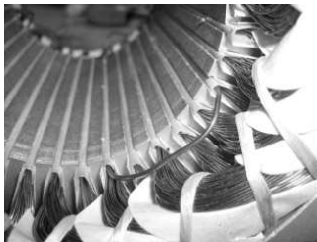
Fig. 10 Stator of rewound PMSM with additional turns (only one can be seen in the figure)
