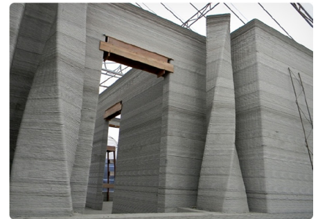
f) vertically printed, in-situ walls and columns. Image: courtesy of Andrey Rudenko, Total Kustom, USA
