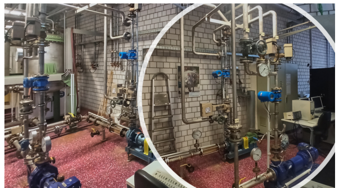
Fig. 1. Pump station used in the lecture Pumps and Compressors in Mannheim University of Applied Sciences.
