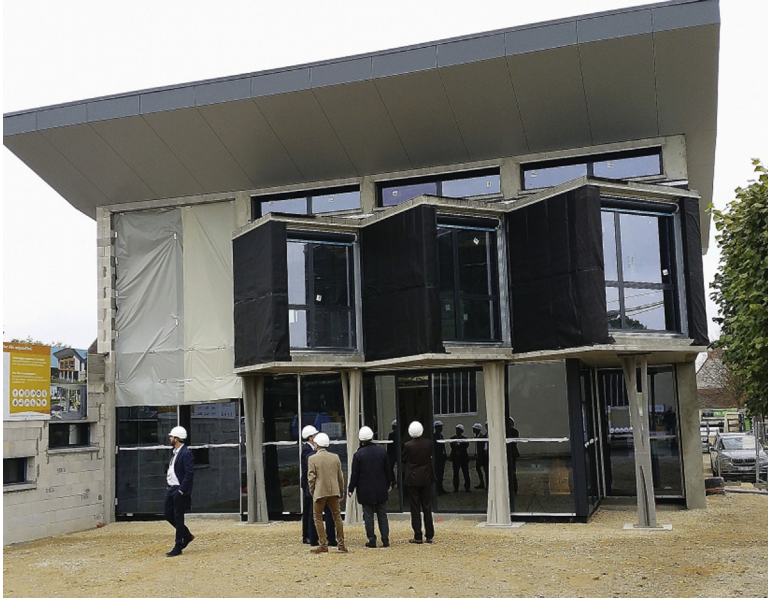
Figure 3.12 Exterior pillars supporting part of the upper floor on the YRYS Concept house in Alençon, France.
