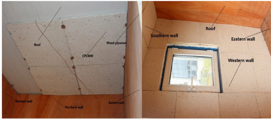
Fig. 13. cPCM wallboards installed on the ceiling and walls of the test cell [121]. Copyright (2019), with permission from Elsevier.
